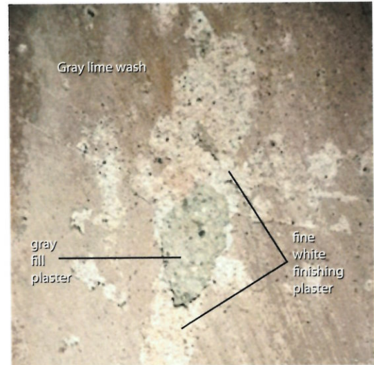
FIGURE 2.26. Flaking paint and plaster expose the stratigraphy of the reconstruction plaster in a loss on the east wall: gray lime wash over a thin white plaster covering a thick layer of gray fill plaster.
