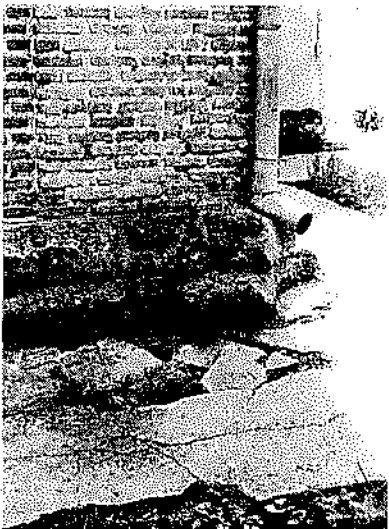
Figure 5. The drainpipe discharges rain water directly onto the concrete pavement at the southwest corner of the narthex at the church in Kintsvisi. (Photo: Nana Kuprashvili)
