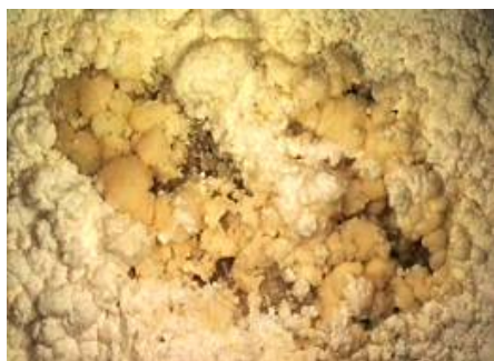
Fig. 2 Spherical formations due to salt efflorescence.
