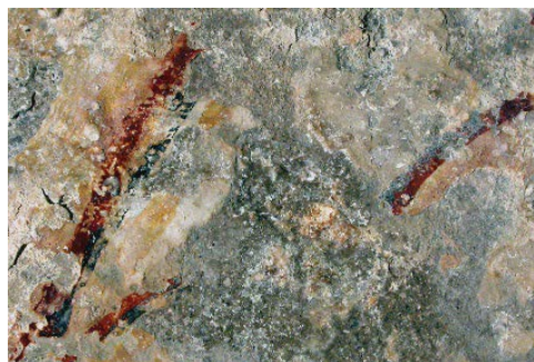
Fig.5 a and b Carbonate deposits before and after removal.
